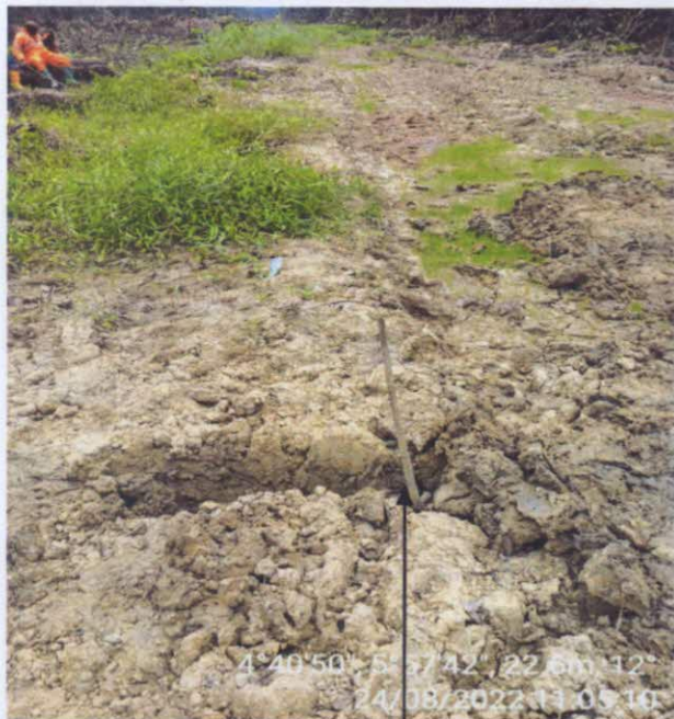
SPILL POINT BEFORE EXCAVATION
